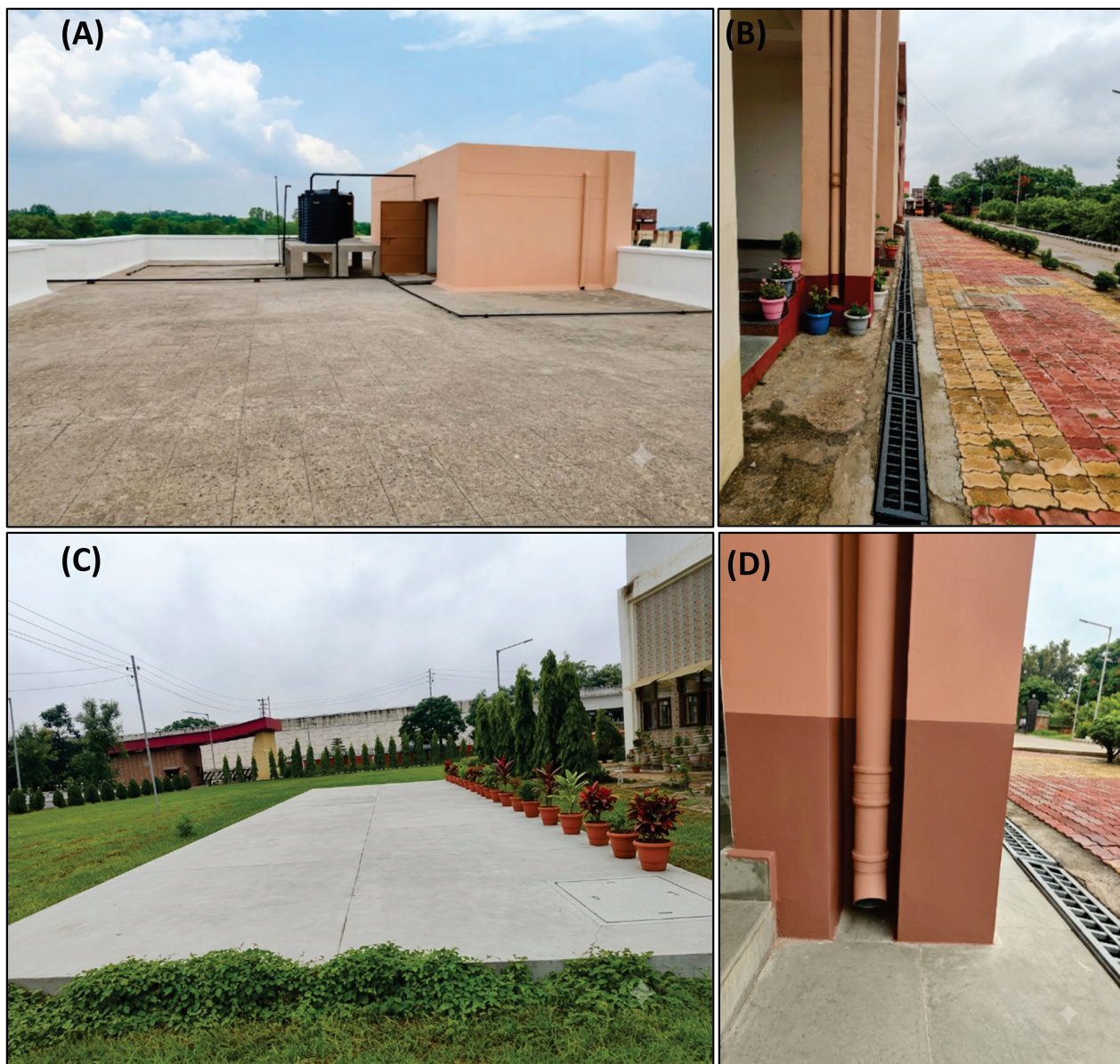
Figure 8.3. Office building rooftop rainwater harvesting and storage system showing (A) rooftop catchment, (B) PVC gutters, (C) downpipes, and (D) storage tank at ICAR-MGIFRI, Piprakothi. Source: ICAR-MGIFRI
