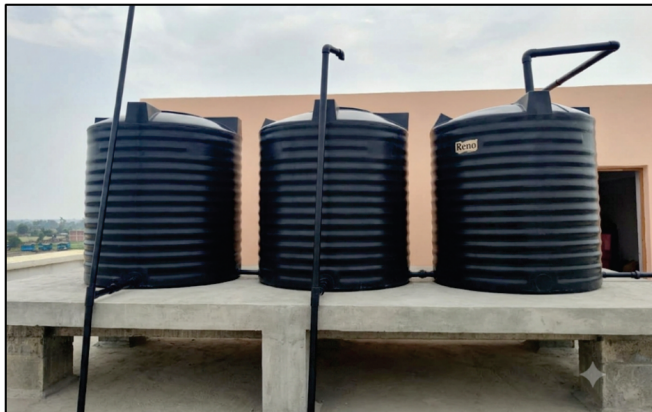
Figure 4.1. Above-Ground Rainwater Storage Tank for temporary storage and utilization of harvested rainwater. Source: ICAR-MGIFRI.
