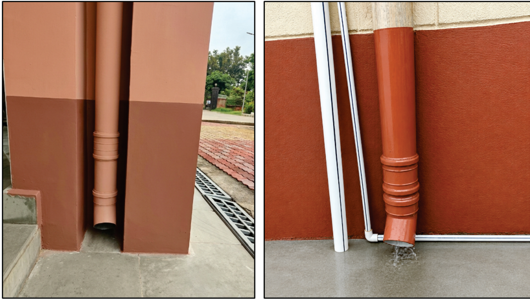
Figure 3.2. PVC conduit (downpipe) for rainwater conveyance. Source: ICAR-MGIFRI.
