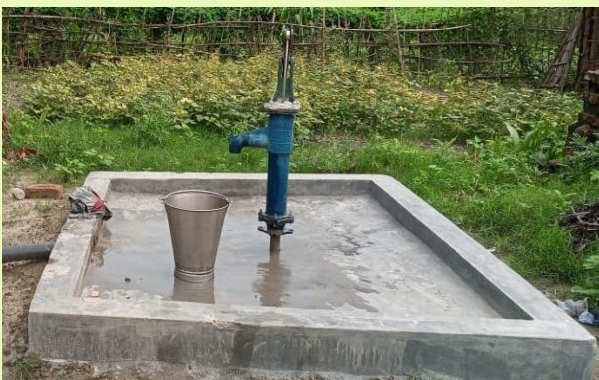
Borewell & handpump at Mahuawa
