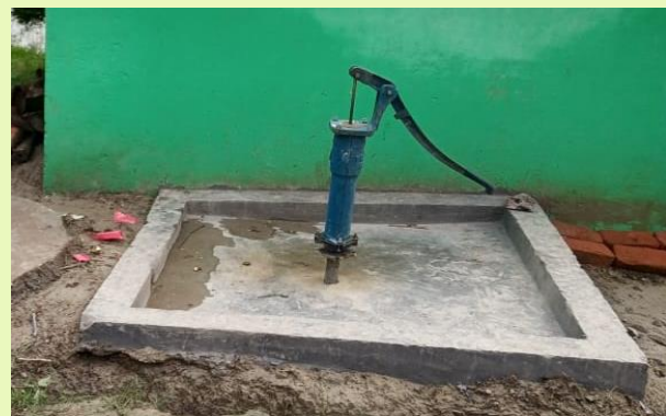
Borewell & handpump at Mahuawa
