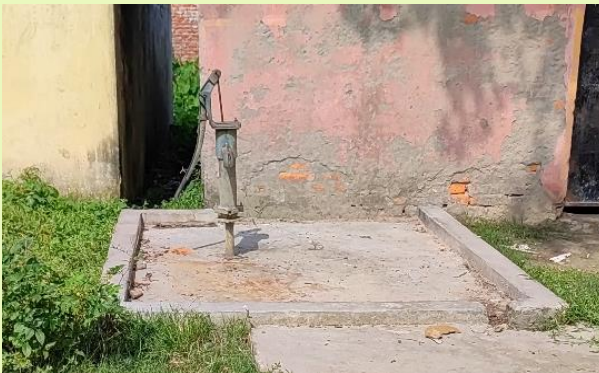
Borewell & handpump at Chandrahiya
